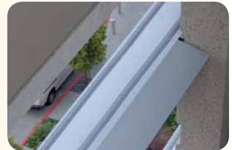
These decorative fins were a favorite roost for about 100 pigeons. Two rows of Flex-Track cleared them off.
