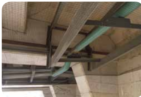
The pipes and beams on the underside of this bridge are sealed off by StealthNet.
